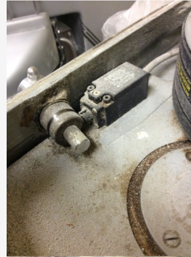
Limit switch requires adjustment
