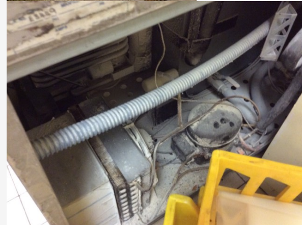
Compressor not working
